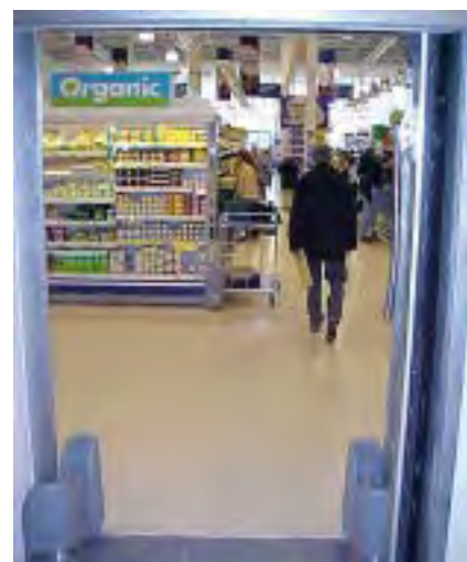
Colt Firepath fire curtains installed at Tesco's in Glasgow. These are designed to separate the main shopping area from the storage area.
