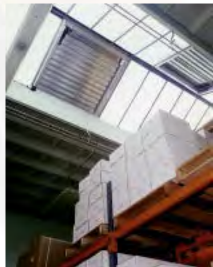
Colt Seefire ventilators installed into glazing at high level.
