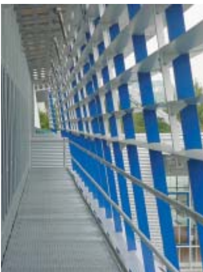
BMW Education & Production Centre, Germany. Over 1000m 2 of controllable solarfin controlled by CCS 2000 was installed along the front façades.
