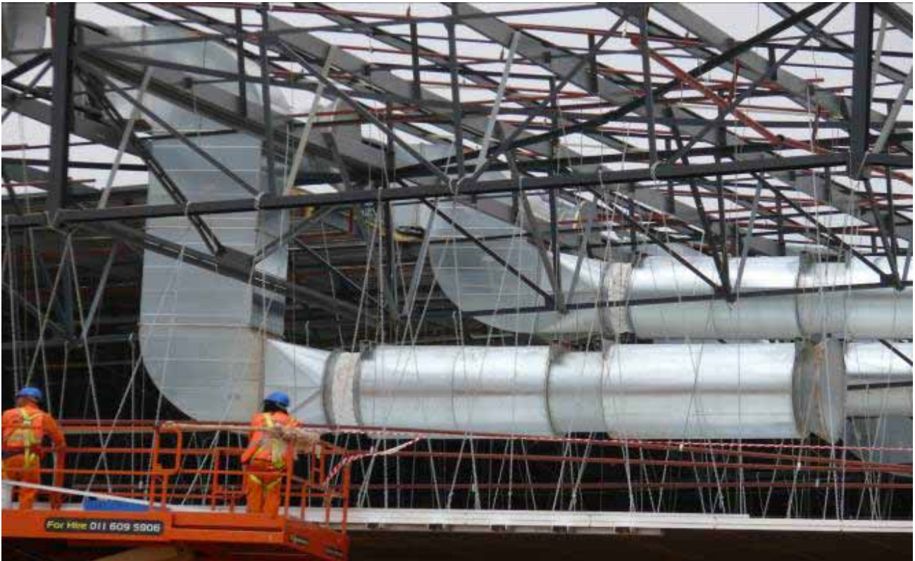
Project: Design, Supply, Delivery & Installation of Dual Purpose Mechanical Smoke Extraction and Day to day Ventilation System Location: Pick n Pay Distribution Centre, Gauteng
