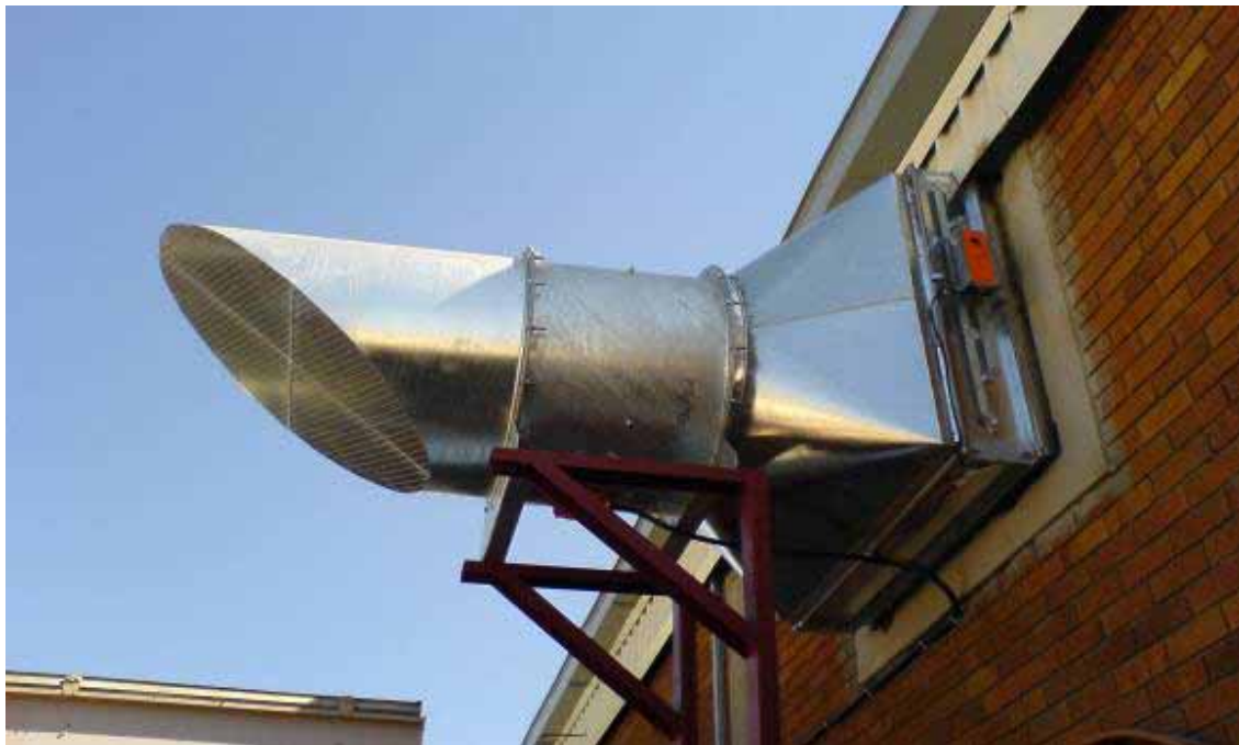
Project: Design, Supply, Delivery & Installation of Mechanical Smoke Extraction System Location: Meltz store Centurion
