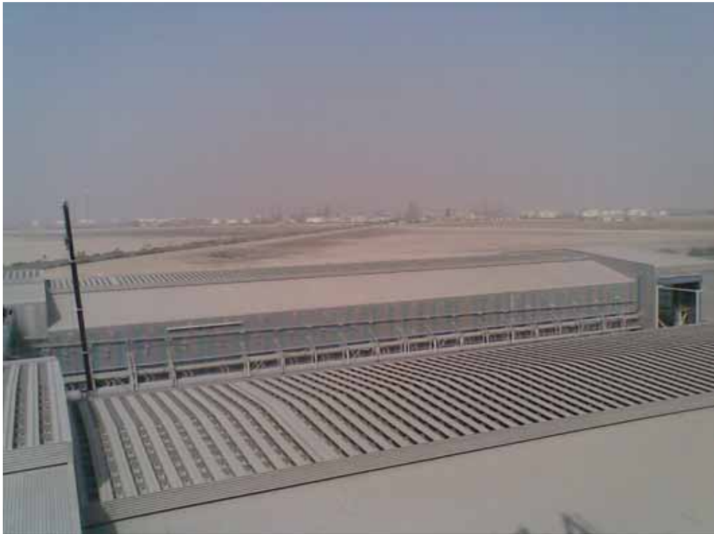
Project: Design, Supply, Delivery & Installation of 51 030 m 2 of Robertson SF 1000 Continuous Ventilator and 325 000 m 2 of A7 Wall and Roof Cladding Location: Oatalum - Qatar
