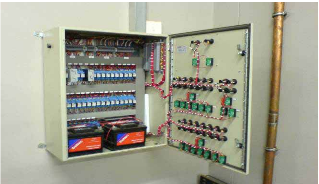
Project: Design, Supply, Delivery & Installation of Smoke Ventilation System Electric Control & Reticulation.
