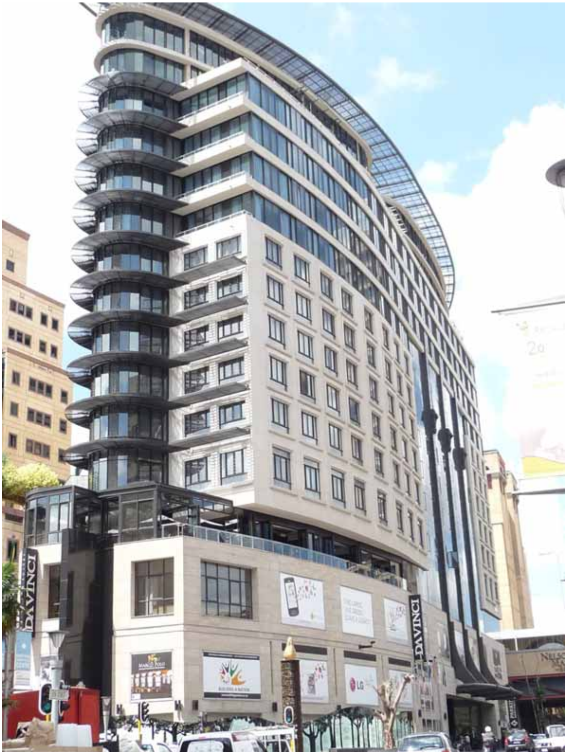
Project: Design, Supply, Delivery & Installation of Colt Solar C Series Screening Louvre System - Location: Legacy Corner, Sandton
