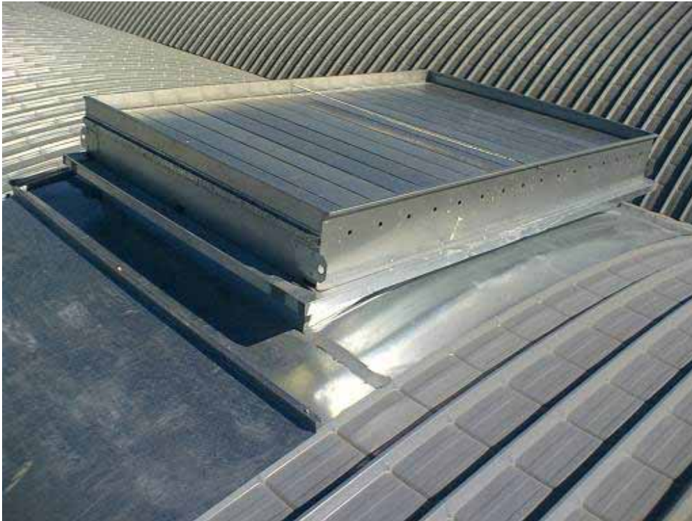
Project: Design, Supply, Delivery & Installation of Electrically Operated Roof Ventilators Location: Middestad Mall
